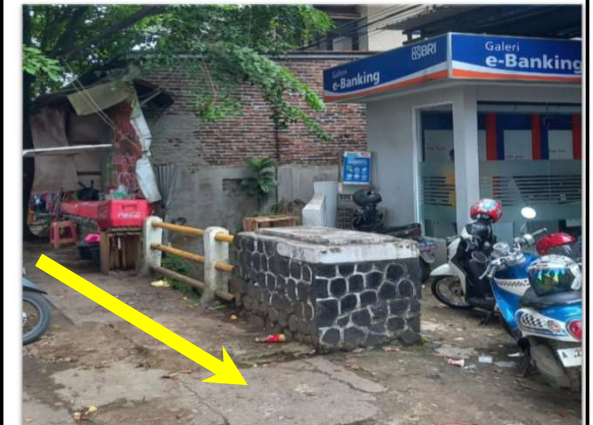
Lokasi Rencana JDU Crossing Drainase Pipa HDPE SDR 17/PN 10 ND Ø 6 "(Drainase Sunangiri- HDD)
